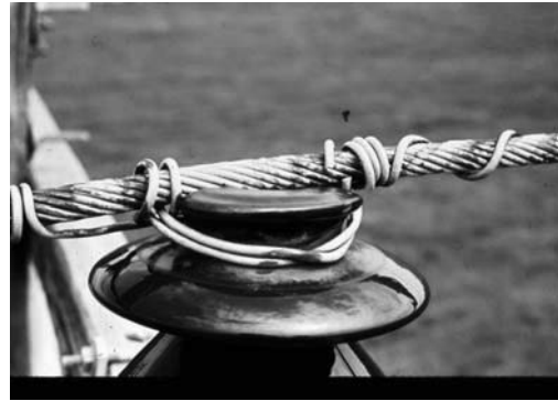
Figure 5 – Abrasion Damage at Loose Hand Tie
