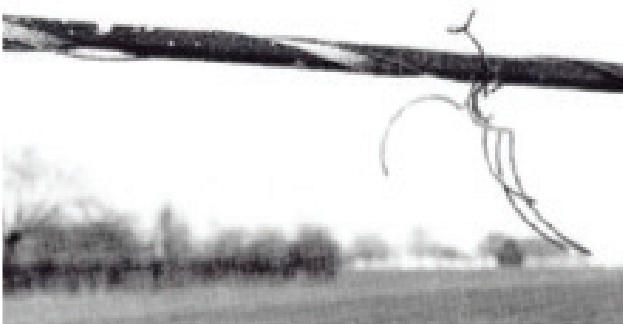
Figure 16: Conductor Damage due to flashover (Leppers, P. H., 1981).
