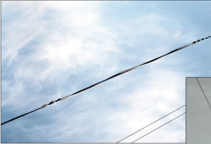
Air Flow Spoiler as seen in the field.
