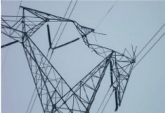
Figure 20: Structure damage due to galloping
