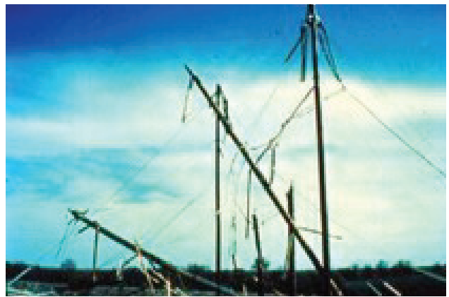
Figure 19: Structure damage due to galloping
