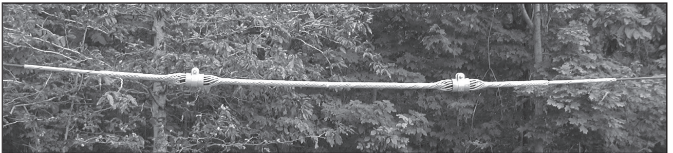
FIGURE 30: FIBERLIGN SPREAD DOUBLE SUSPENSION ON ADSS CABLE
