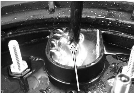
Leak occurring at the cable entry of the grommet
