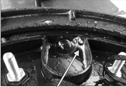
Leak occurring at the corner of the cable port
